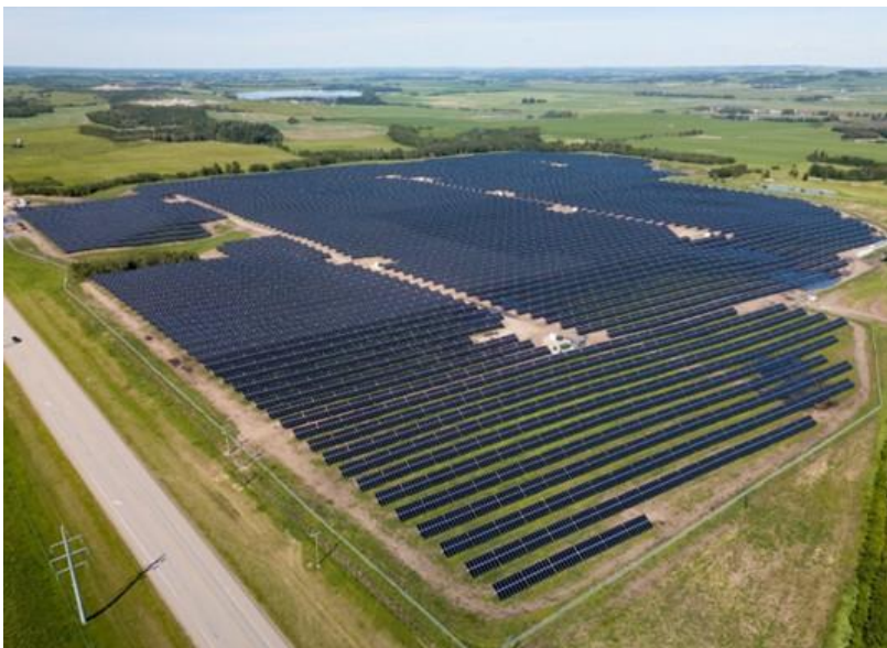
Elemental Energy Inc. Innisfail Solar Farm
