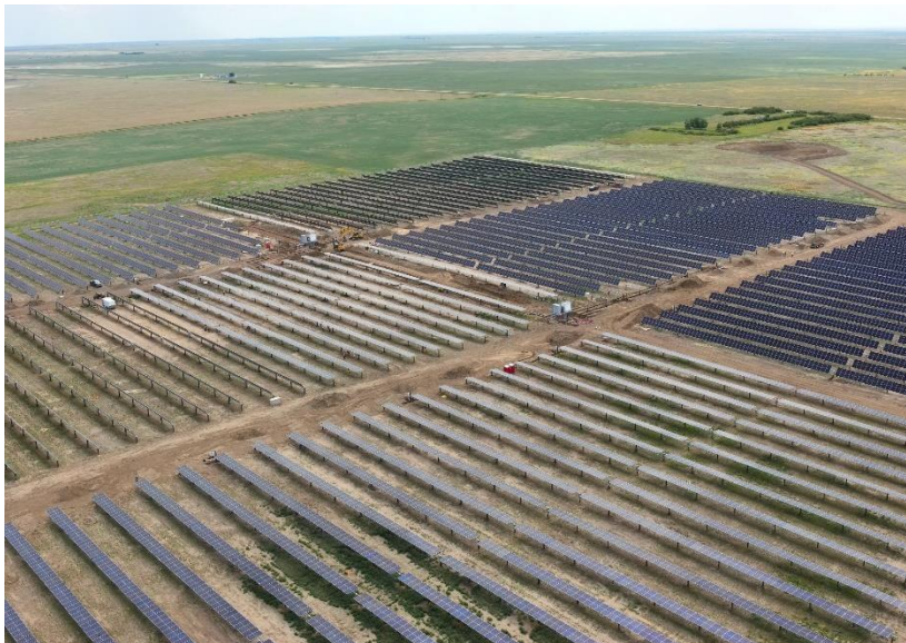
Elemental Energy Inc. Innisfail Solar Farm
